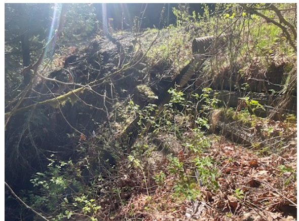
Foundation appears to be cast over fill which is eroding.
