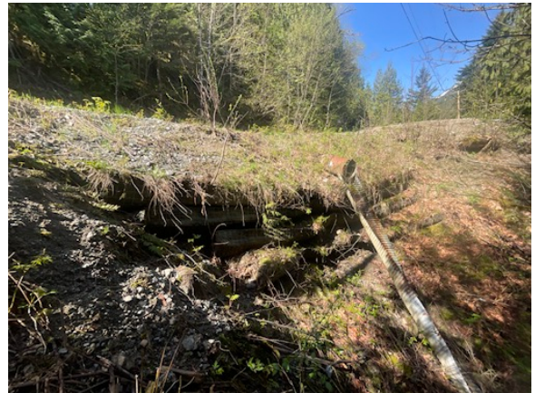
CMP outlet making water, but all elements of wall have failed. Each layer of mesh has failed as well as the whole foundation causing significant sagging in the middle
