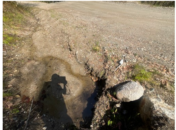
CMP Inlet plugged
